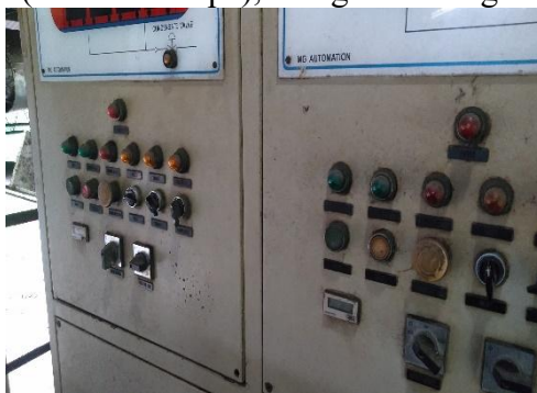
Figure 6. Indicator Lights and Siren
